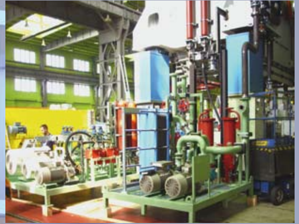
Pressure supply stations for cooling and lubrication
