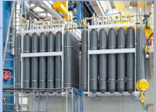
Nitrogen bottle stations built onto the side as a back-up for piston accumulators
